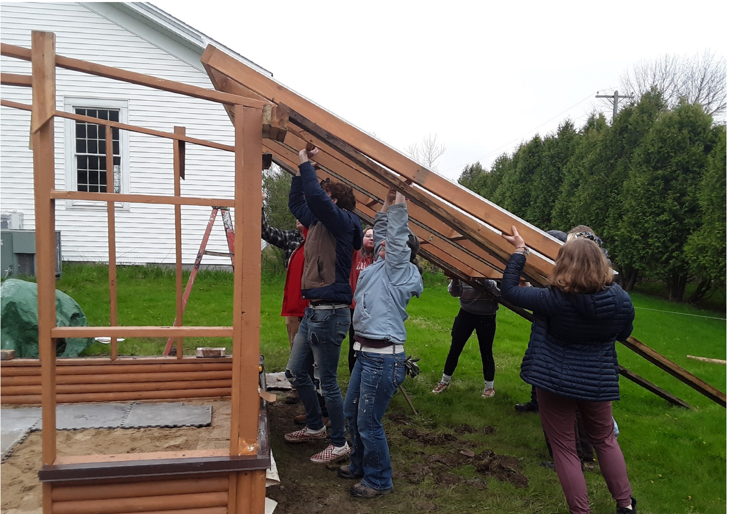
Seniors and staff work together to complete the difficult task of raising the roof of the sunroom the seniors chose to build.
